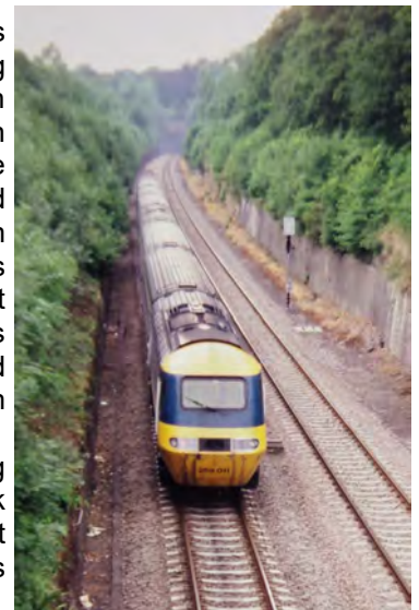
Down HST about to enter Box Tunnel. Note the cutting wall on the left with tree growth
